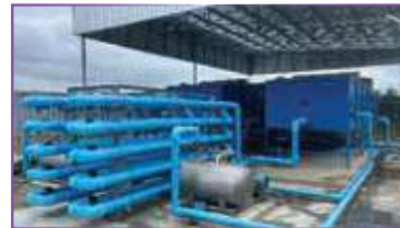
2. DAF Dissolved Air floatation System
