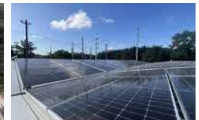
Solar rooftop at factory's Trang Branch
