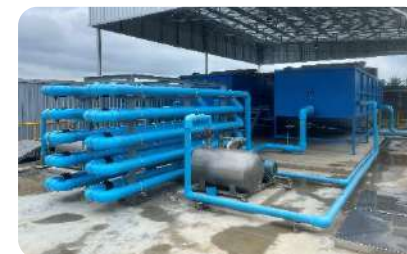
2. DAF Dissolved Air floatation System
