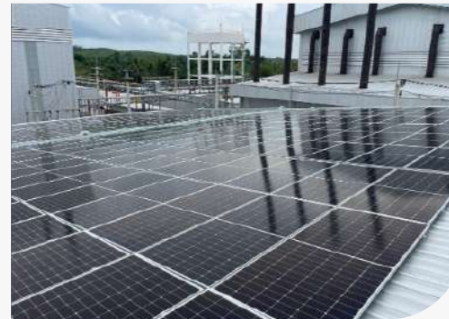
Solar rooftop at factory's Sadao P.S. Branch
