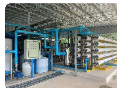
4. RO Machine Unit
